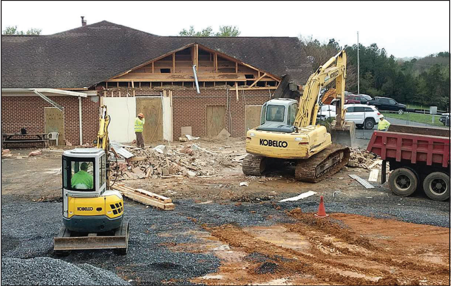
WORKERS demolish the former conference room and kitchen of the Rockbridge Area Health Center last week in preparation for the start of the center's expansion project. (Matt Paxton photo)
